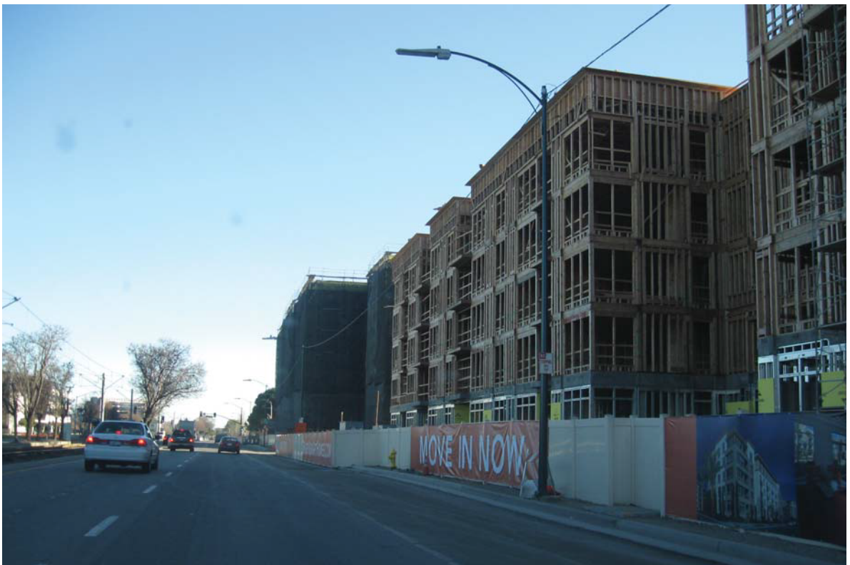
PHOTO 2: Southbound N. 1st Street, near the N. 1st Street/River Oaks Parkway intersection.
