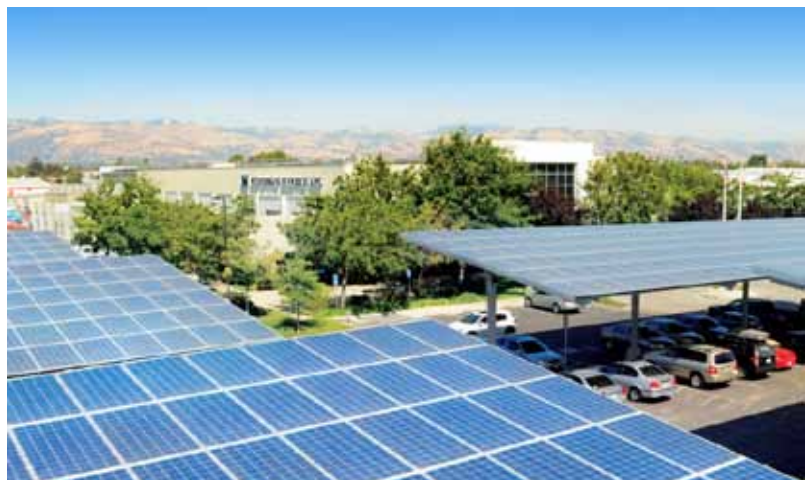
Cupertino Electric’s Solar Demonstration
