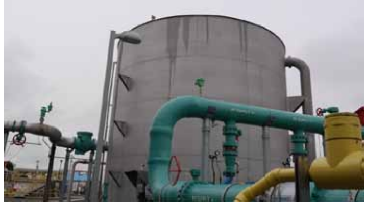
Purified water storage at the Silicon Valley Advanced Water Purification Center
