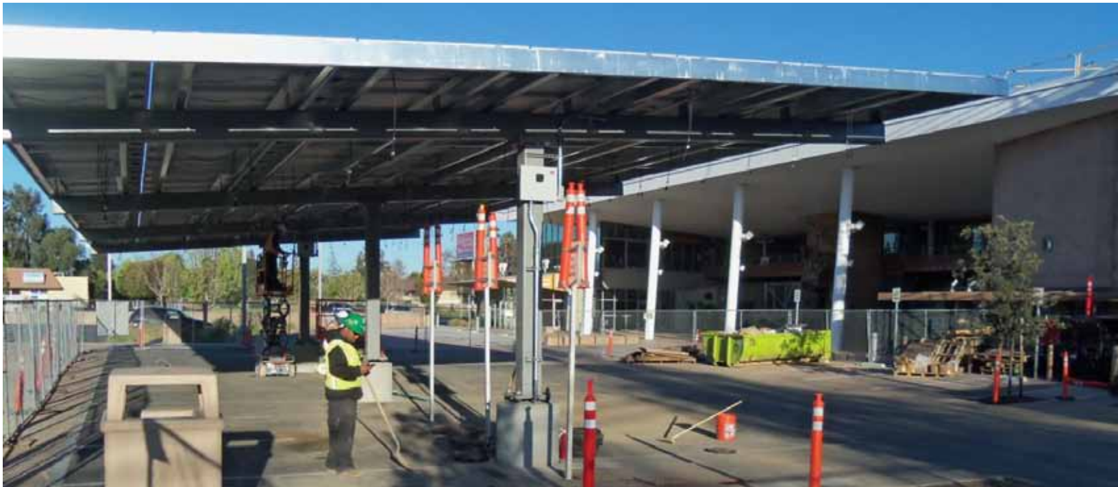
Bascom Library and Community Center Solar Installation completed April 2014.
