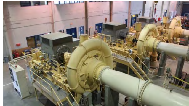
Electric Blowers in Building 40
