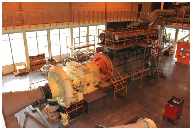
Engine-driven Blower in Secondary Blower Building
