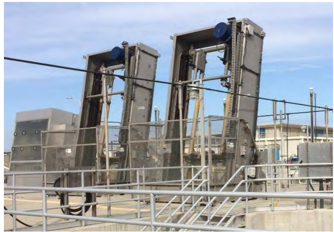
Headworks 1 Bar Screens
