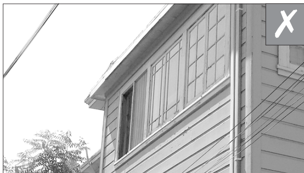
If window replacement is necessary, then all windows being replaced should be the same style as those seen historically.
