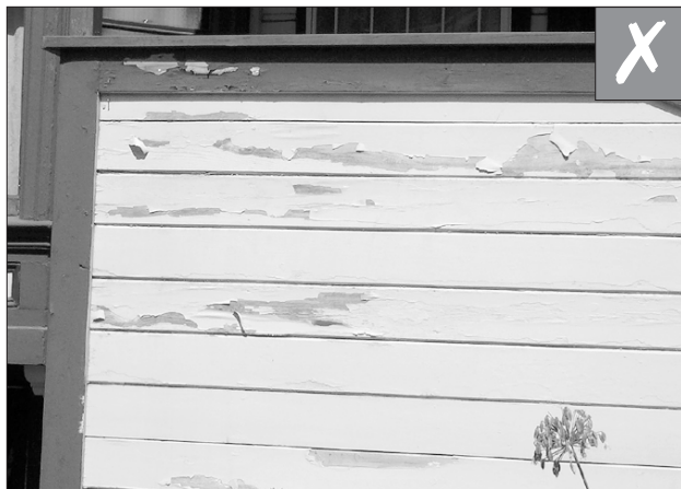
Prior to painting, remove damaged or deteriorated paint only to the next intact layer, using the gentlest method possible.
