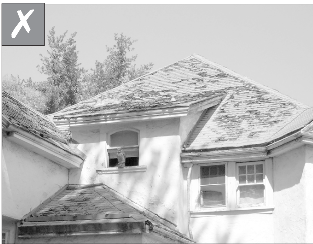
Roof materials are the most susceptible to deterioration, and their replacement may become necessary in time.
