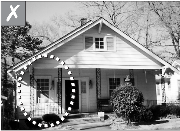
This porch has experienced an inappropriate alteration; wrought iron supports have replaced wood piers. Compare it with its “twin” in the photo below. (Spartanburg, SC)
