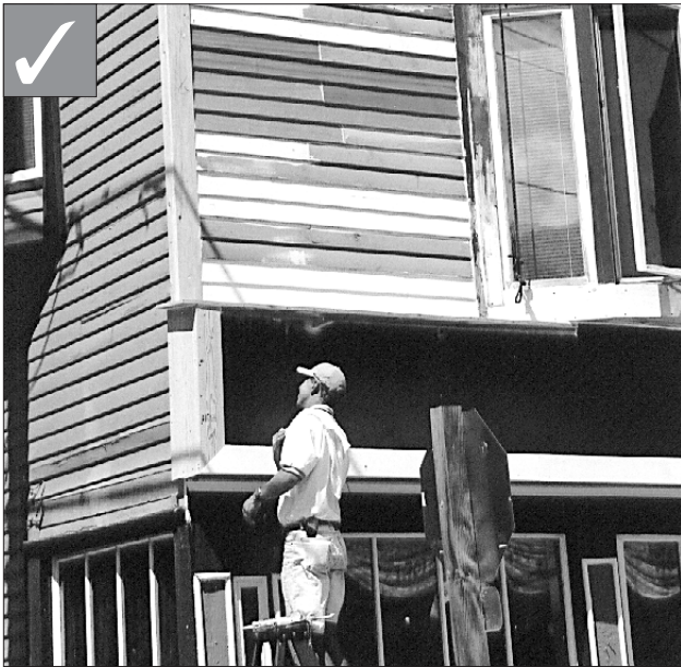
Repair wood features by patching or piecing-in new wood elements that match the original.
