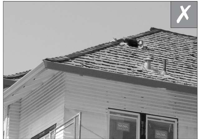
Look for breaks, or holes in the roof surface, and to check the flashing for open seams.
