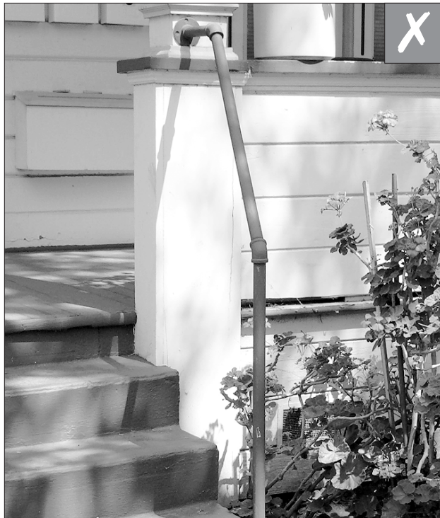
While a simple design solution, the use of metal pipes as replacement porch rails is inappropriate.
