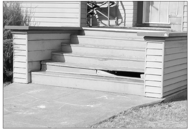
Repair those elements of a porch that are deteriorated.
