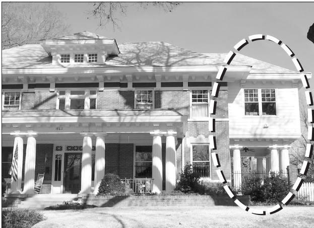
A more recent addition that is not historically significant may be removed. (Memphis, TN)
