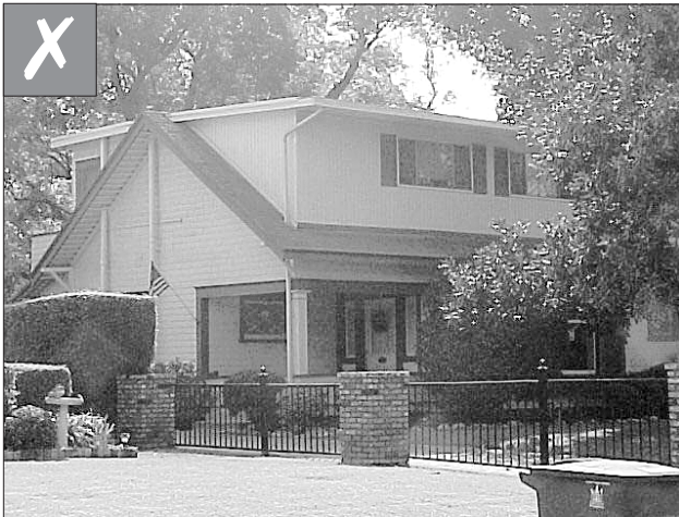
A new dormer should remain subordinate to the historic roof in size and character. The dormers on the front and rear of this structure are too large and are inappropriate.
