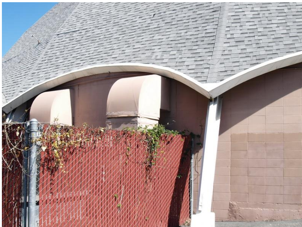
Ventilation system located behind main dome.
