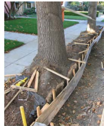
Illegal and improper root pruning can kill a tree or cause it to fail.
