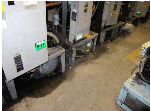
Photograph 8. View staining on concrete below condensing units.
