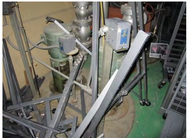
Photograph 16. Sanitary sewer lift station in Sports Authority basement.
