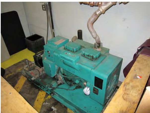
Photograph 9. Natural gas fueled generator in Safeway.
