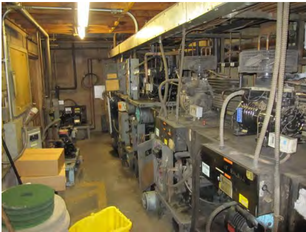
Photograph 7. Condensing units in Safeway "Motor Room."
