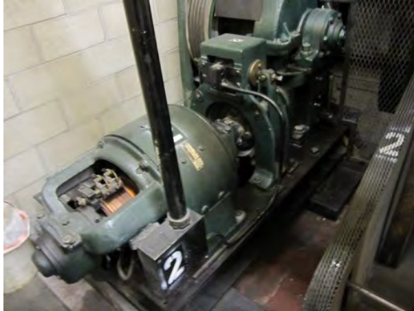
Photograph 17. Electric elevator motor in Sports Authority basement.
