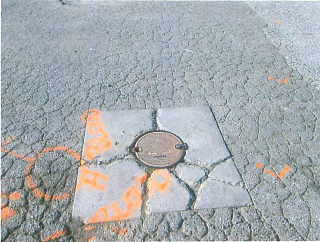
Photo 5: Looking at one of the existing groundwater monitoring wells
