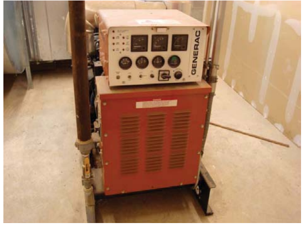
26. Natural gas-powered generator on the mezzanine of Building 1.
