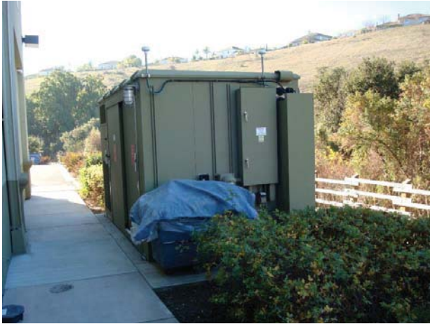
19. View of the cell phone tower equipment for Nextel at the western side of the subject property.
