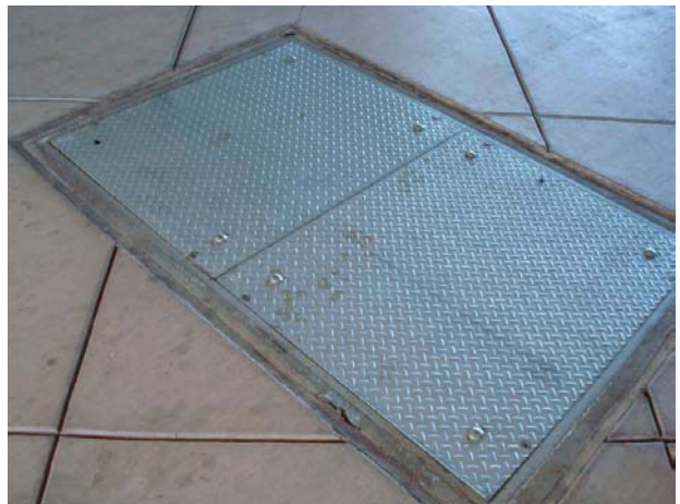
10. Electrical conduit pull box at the central breezeway within Building 2.
