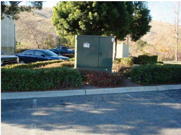
17. View of a pad-mounted transformer.
