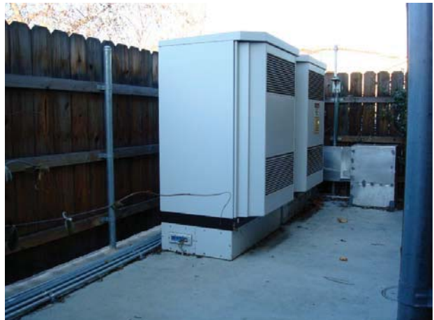
18. View of the cell phone tower equipment for T-Mobile at the western side of the property.
