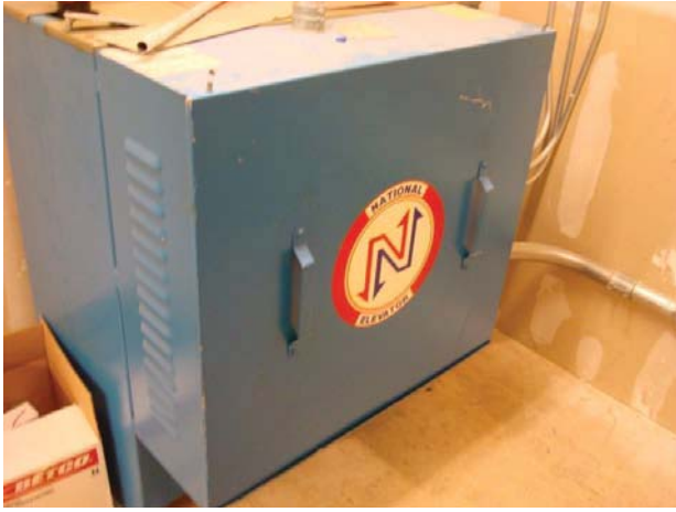
25. Elevator equipment within Building 1.
