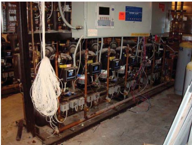
27. Compressors for refrigerators on the mezzanine of Building 1.
