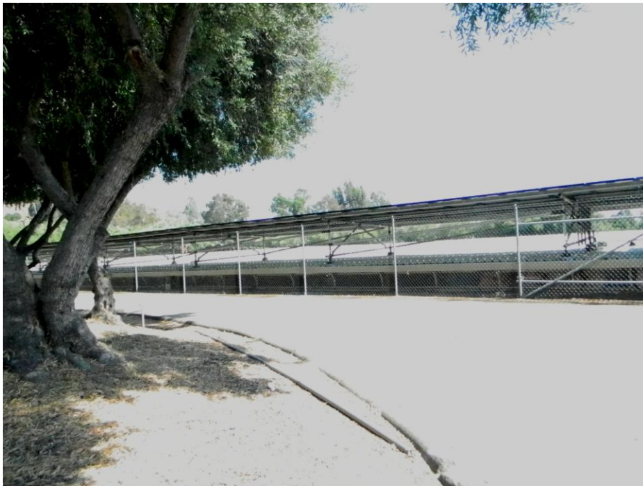
Figure 6 Solar modules along north elevation of the Columbine Reservoir roof
