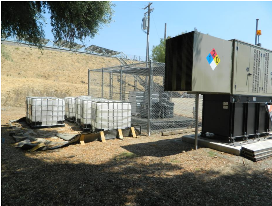
Figure 12. Mechanical and storage area, facing southeast
