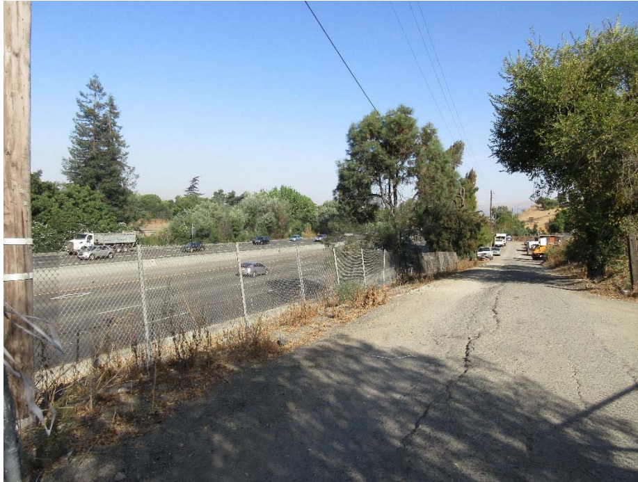
Photo 3: The on-site access road, looking north from the southern area of the project development footprint
