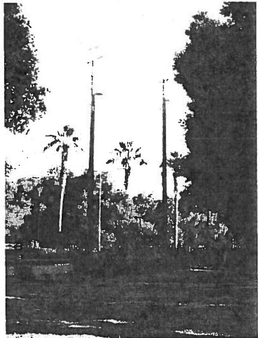
POLE MOUNTED TRANSFORMERS
