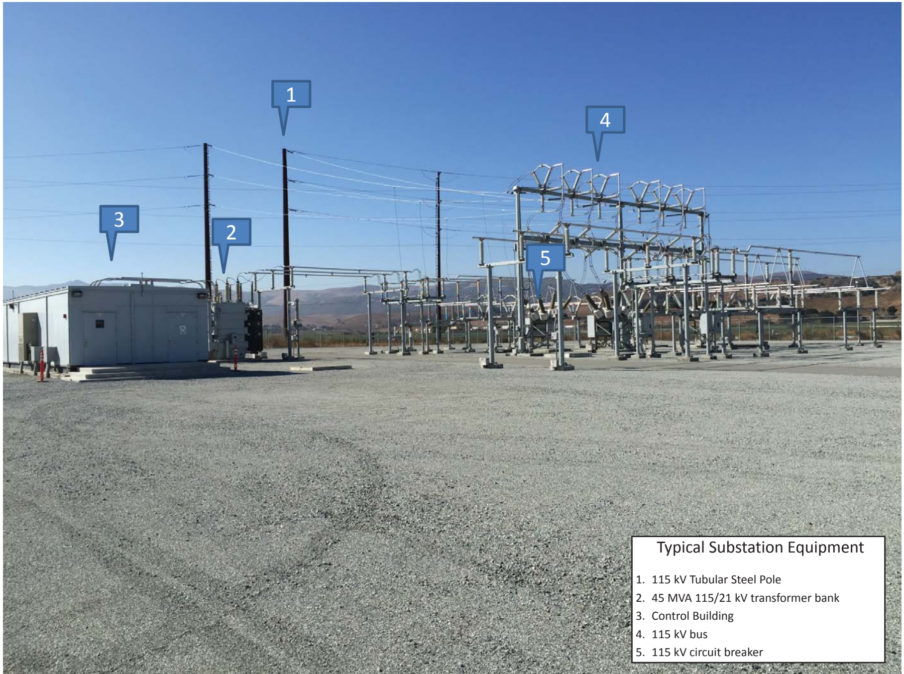
PHOTOGRAPH OF TYPICAL SUBSTATION EQUIPMENT
