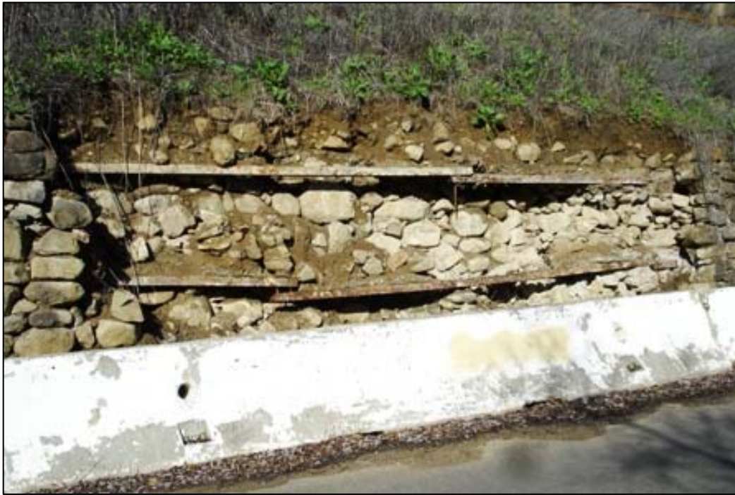
Damaged sections of masonry retaining wall along Penitencia Creek Road. View NE. Note use of former railroad rails as reinforcement.
