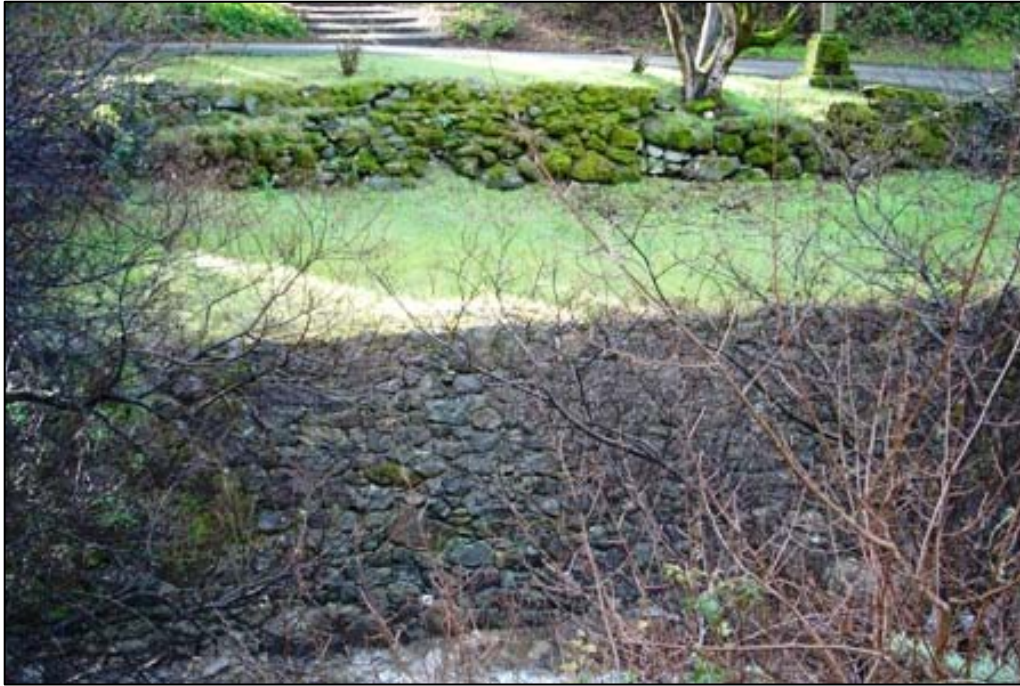
Masonry Wall along Penitencia Creek near Automobile Bridge 4 and Log Cabin picnic area. View to the south.
