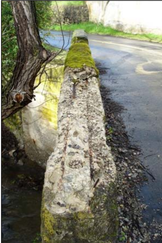
Northwest view of damaged railing.
