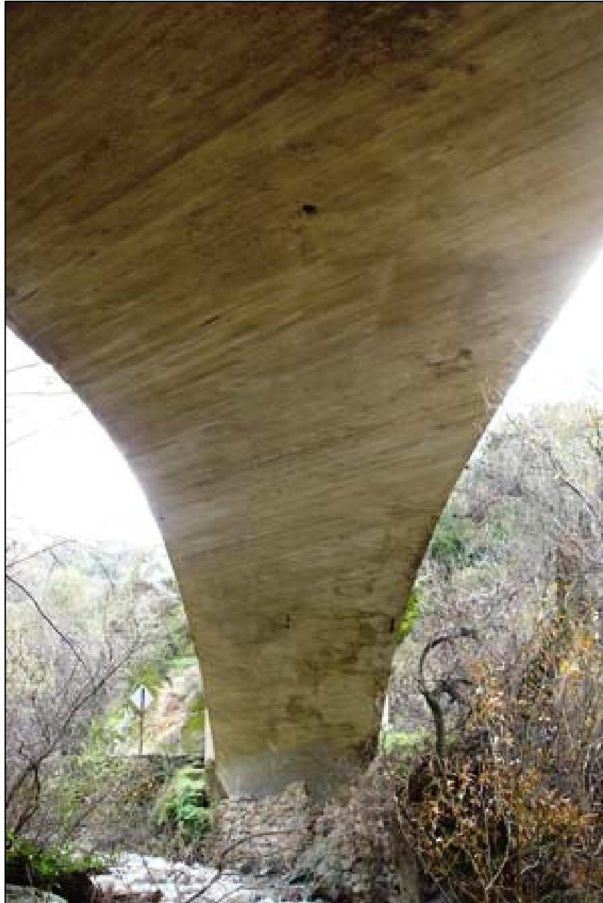
Pedestrian Bridge 5. Underside of Penitencia Creek arch span. View to the south.
