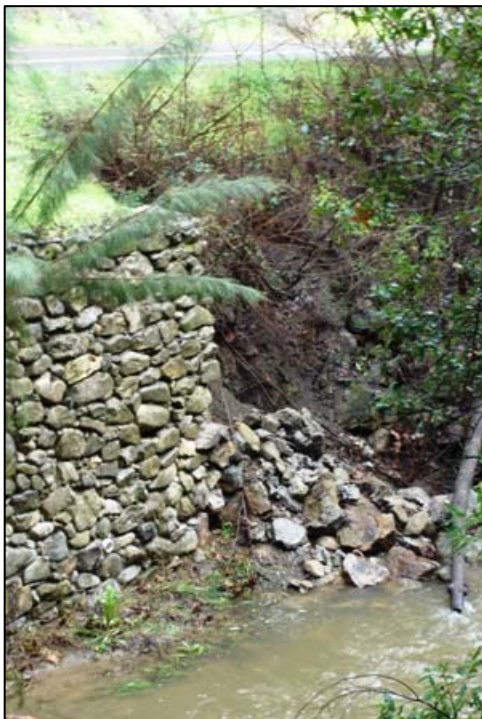
Failing masonry wall, north bank Penitencia Creek Alum Rock Falls Road in background. View Northeast.
