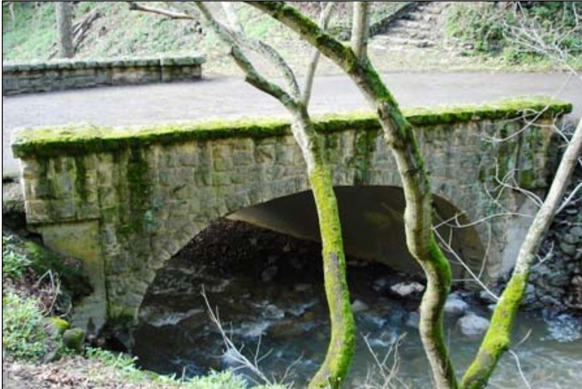
Automobile Bridge 6. View to the NE. Note piece of faux-ashlar finish missing from left abutment.
