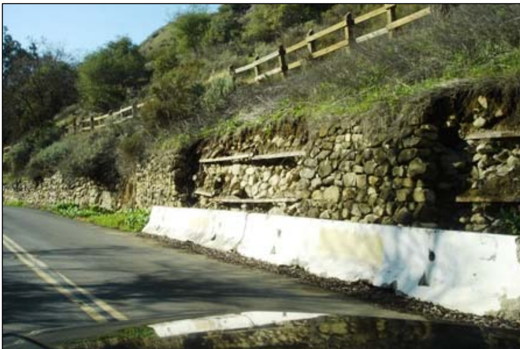
Damaged sections of masonry retaining wall along Penitencia Creek Road. View NW. Note use of former railroad rails as reinforcement.
