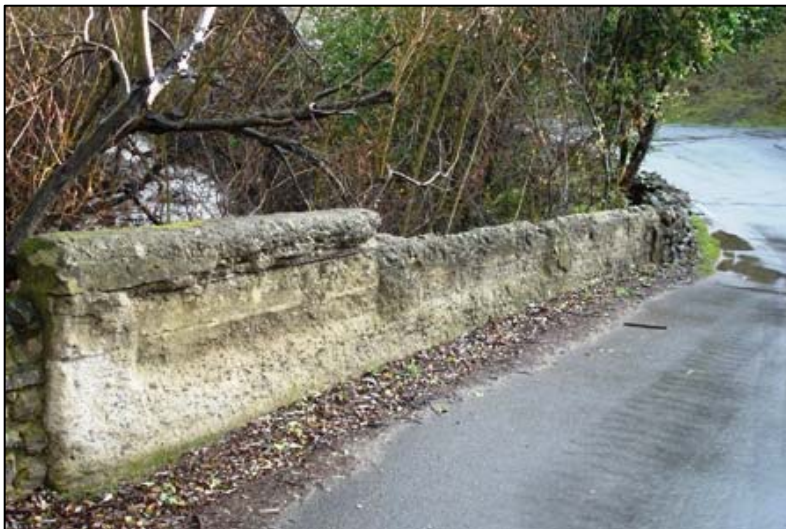
View of damaged railing. View west.
