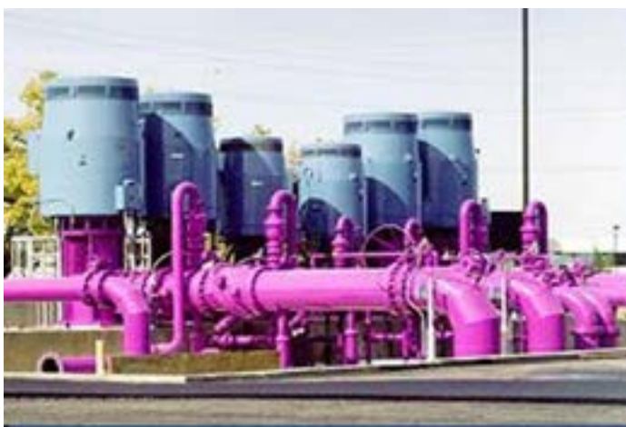
SBWR main pump station
