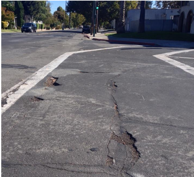
Crossing Shasta Avenue at Park Ave. (District 6), PCI 78, last maintenance in 2002; potholes filled in January 2015
