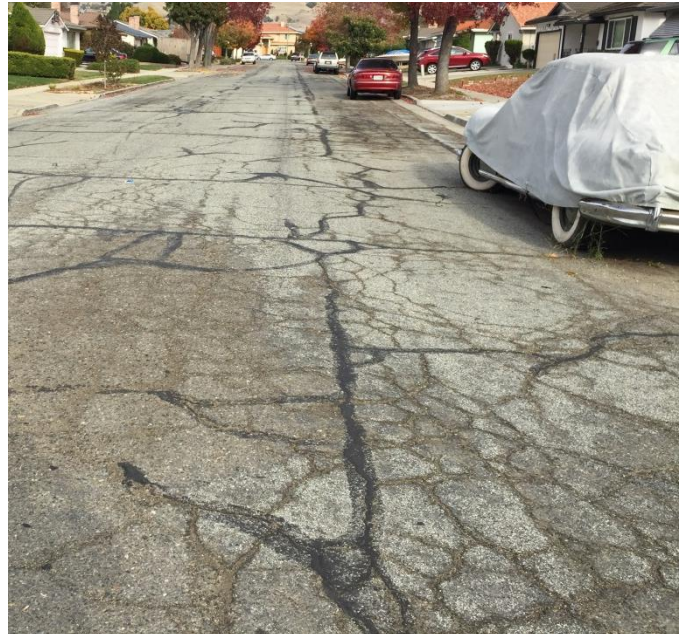
Wilsham Drive (District 4), PCI 18, last maintenance in 1997
