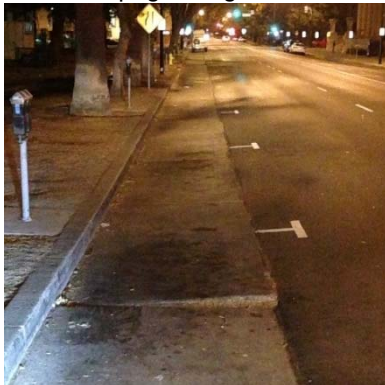
↑ A lifted concrete slab along the Central Business District route during scheduled street sweeping on August 20, 2015.
