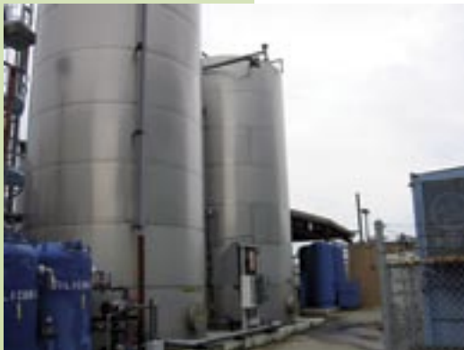
RO reject and backwashes from the RO/DI system flow directly into the reclaim tank. A piping system delivers the reclaimed water to 6 main air scrubbers.
