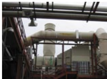
Vishay Siliconix's main air scrubbers accounted for about 15% of the facility's total water use.
