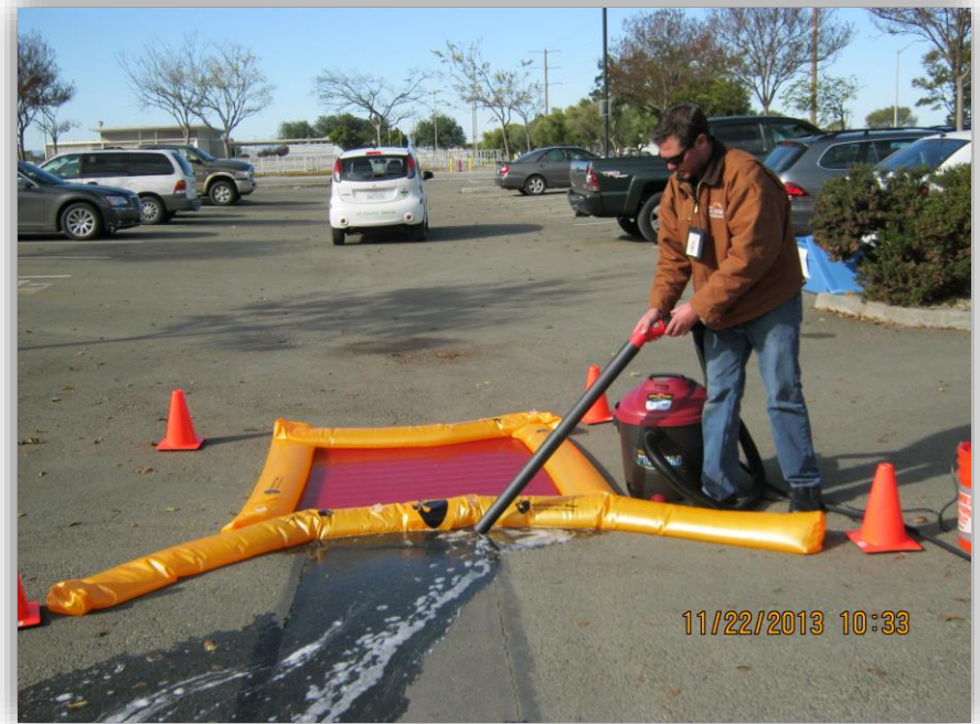
A dry/wet vacuum collecting wastewater. A mat and berms are filled with water to protect a storm drain from runoff.
