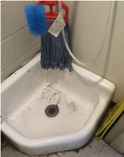
Sanitary sewer drain flows to treatment plant.
