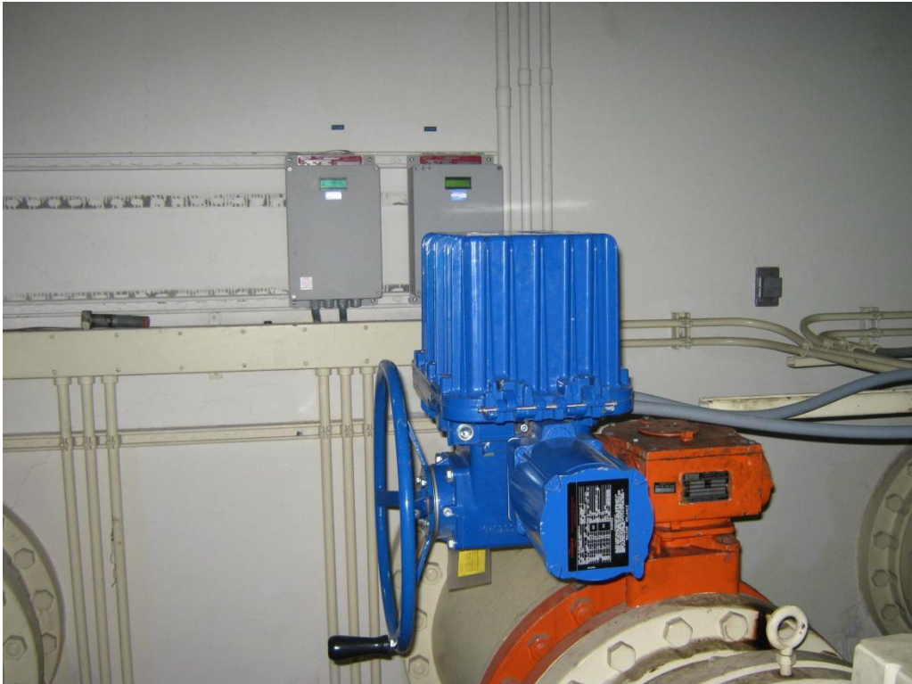
Figure 4: Nitrification Flow Clarifier A-4 Limitorque
