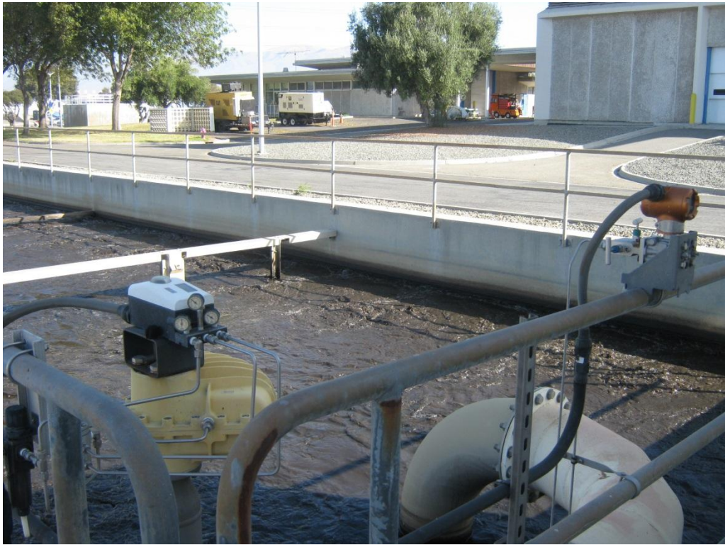
Figure 3: Nitrification Aeration Tank Anaerobic Air Valve
