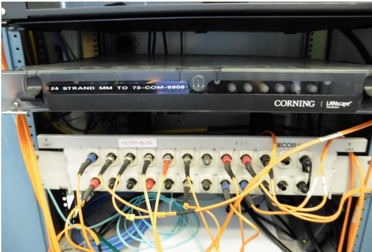
Figure 2 — Fiber Optic Patch Panel at TPS Operations Building
