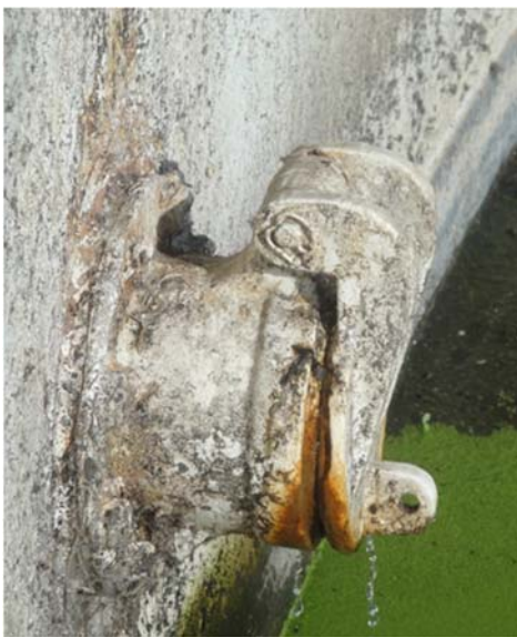
Figure 2 – Inoperable and corroded groundwater relief valve
