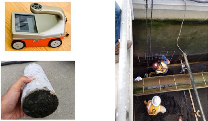
Figure 2: Concrete scanning and coring to evaluate structural conditions in the Filter Block.
