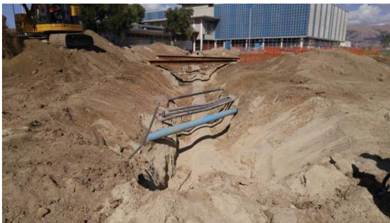
Figure 2: RWF process piping located adjacent to other utilities
