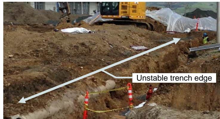
Figure 1: A potentially unstable trench and pipe pose an exposure to injury to the worker in the trench
