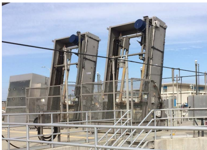
Figure 4: HW2 existing bar screens showing the two single rake bar screens on the right that will be replaced with new multi-rake bar screens, similar to the screen on the left.
