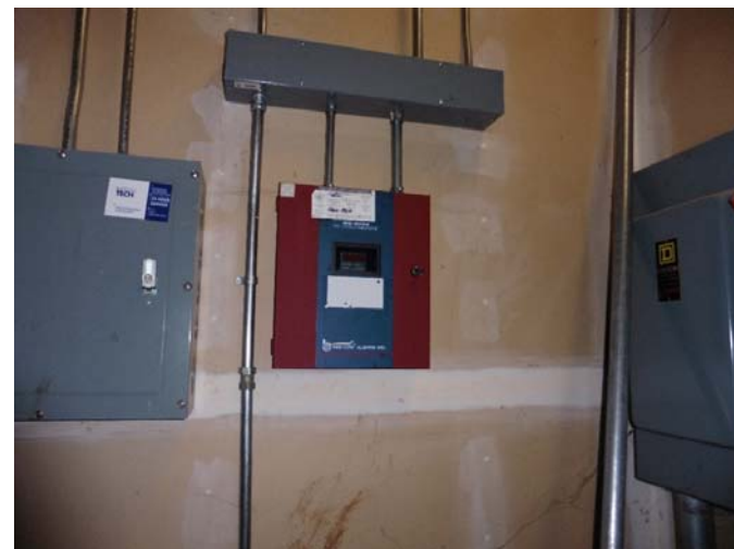
Figure 4: Fire Control and Communicator in CL/SO2 Building
