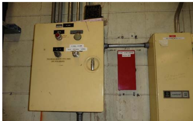
Figure 3: Global Alarm Panel in the Filter Influent Pump Station
