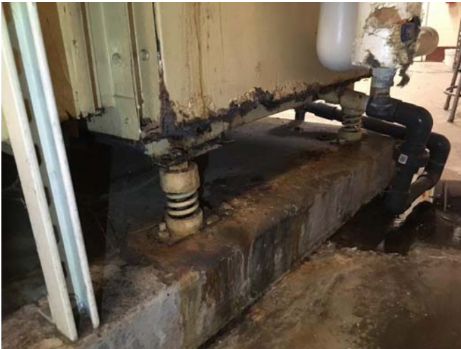
Figure 4: Heavily Corroded Air Handler Unit
