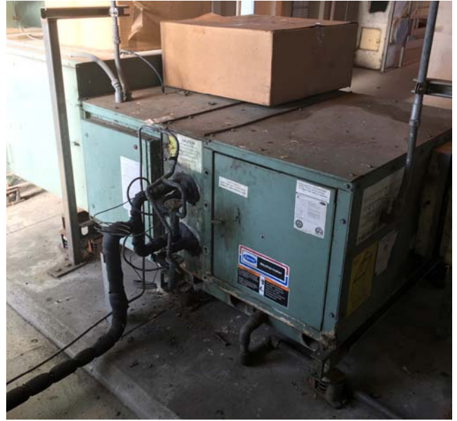
Figure 3: Aging Air Handler Unit
