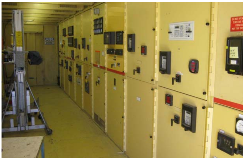
Figure 4: Interior of Existing M4 (5kV) Switchgear Enclosure
