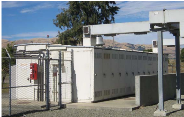
Figure 3: Exterior of Existing M4 (5kV) Switchgear Enclosure
