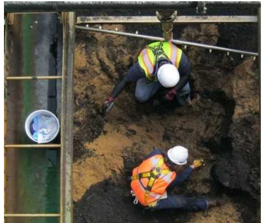
Photo taken during an inspection of filter media. This project will replace filter media and remove the surface wash system.
