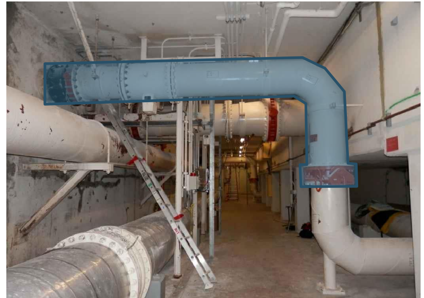
This project will replace 20" valves, meters, and piping in the Nitrification Tunnel.
