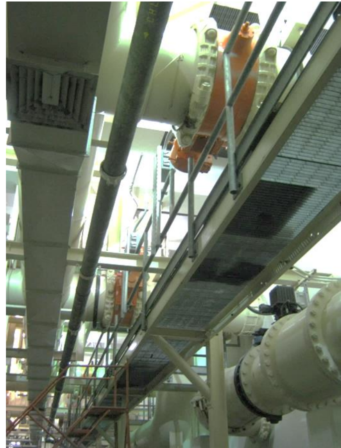
There is limited space for valve replacement in the filter gallery.
