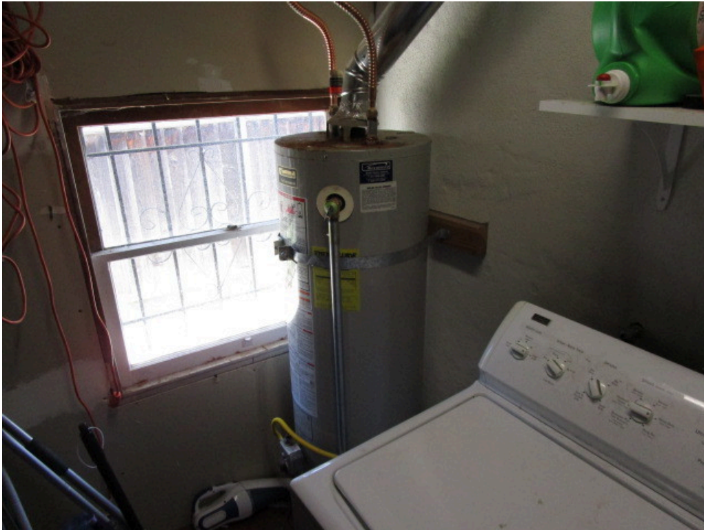
19. 383 South Baywood Avenue residence - water heater
