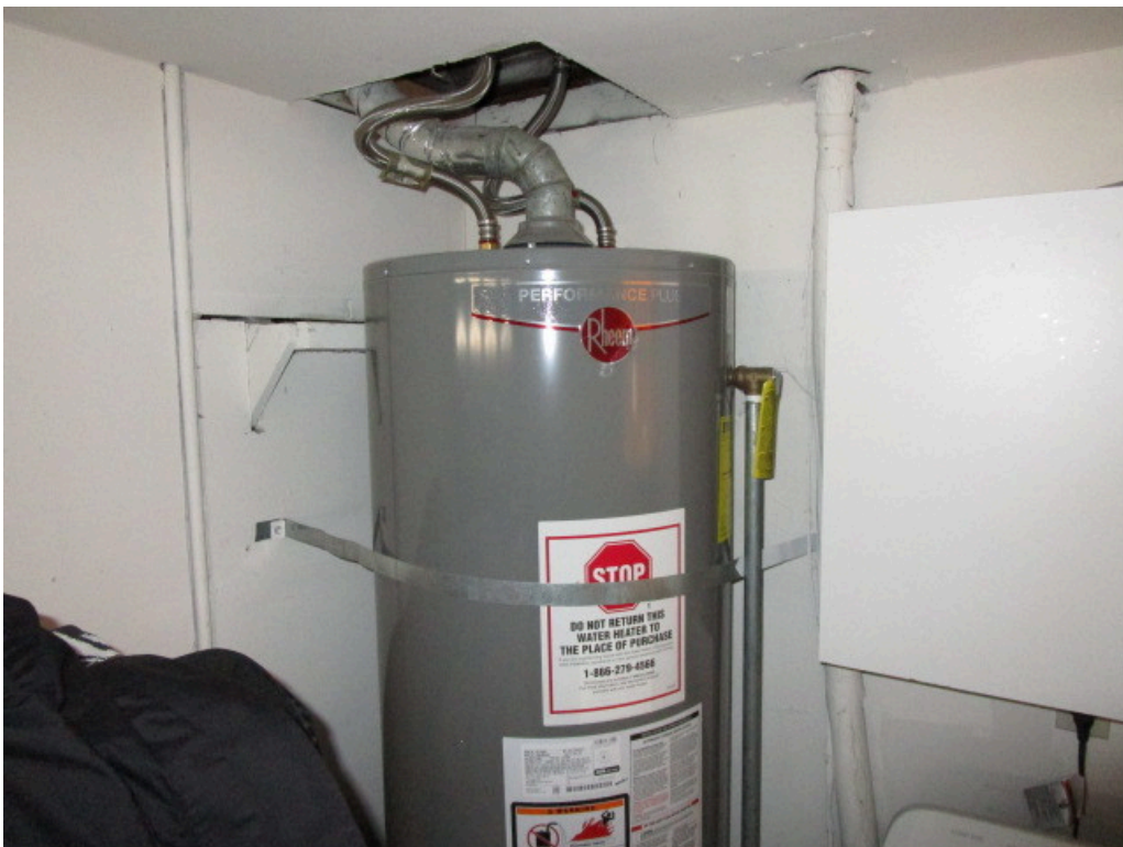
26. 376 South Baywood Avenue - water heater
