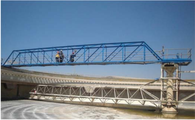
Figure 4: Clarifier Interior and Mechanism
