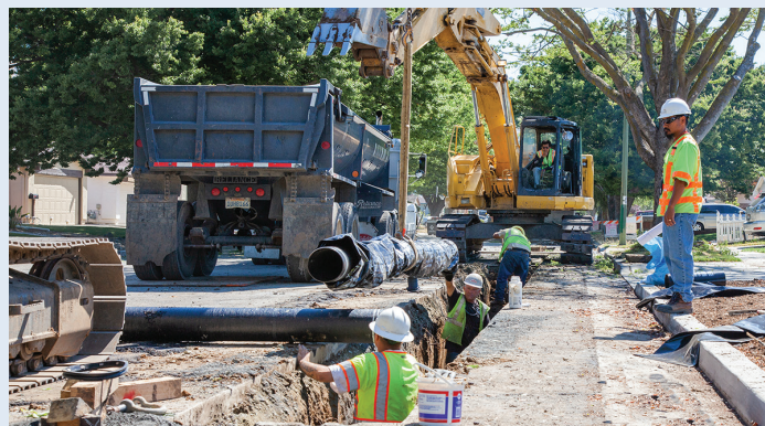
David Bermillo, Principal Construction Inspector, oversees a pipeline replacement project that ensures the safety and reliability of drinking water for our customers. (Photo by A.J. Valdez)
