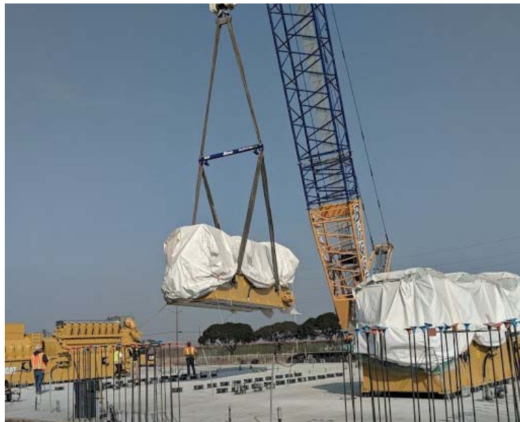
Figure 2: A 330-ton crane was used to set each engine on its base.
