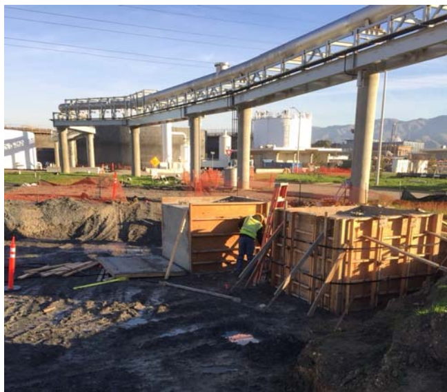
Figure 4: View of pipe rack and new footings, new flare foundation preparatory work.
