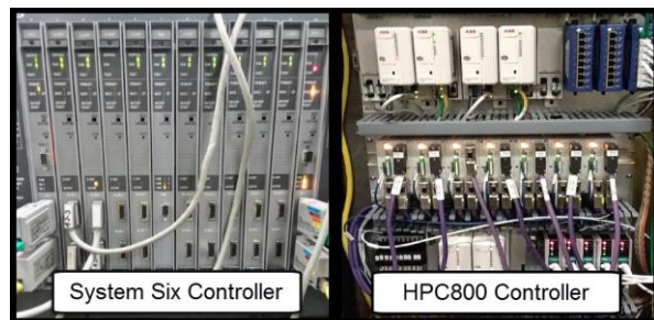
Figure 3: Old System Six controller (left) and new Harmony controllers (right)
