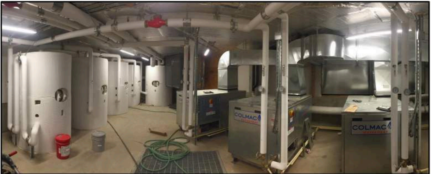
Figure 12: Ecotope Case Study "RCC" system for 194 unit Multifamily building, using best practices in central heat pumps for domestic hot water, from ACEEE presentation by Shawn Oram. 64
