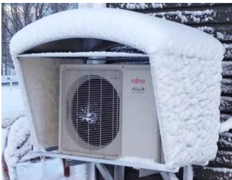
Figure 11: Fujitsu heat pump in the snow (image footnote 62).
