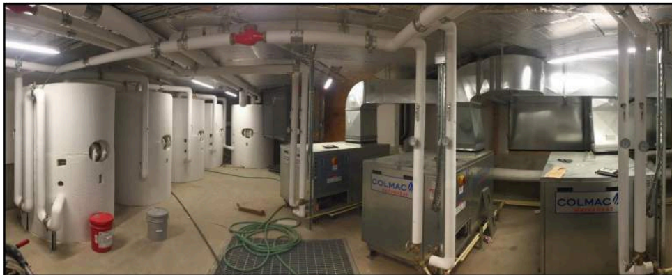
Figure 15: Ecotope Case Study "RCC" system for 194 unit Multifamily building, using best practices in central heat pumps for domestic hot water, from ACEEE presentation by Shawn Oram.
