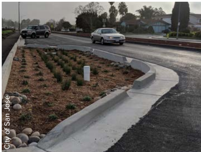
Bioretention Curb Extension on Chynoweth Avenue
