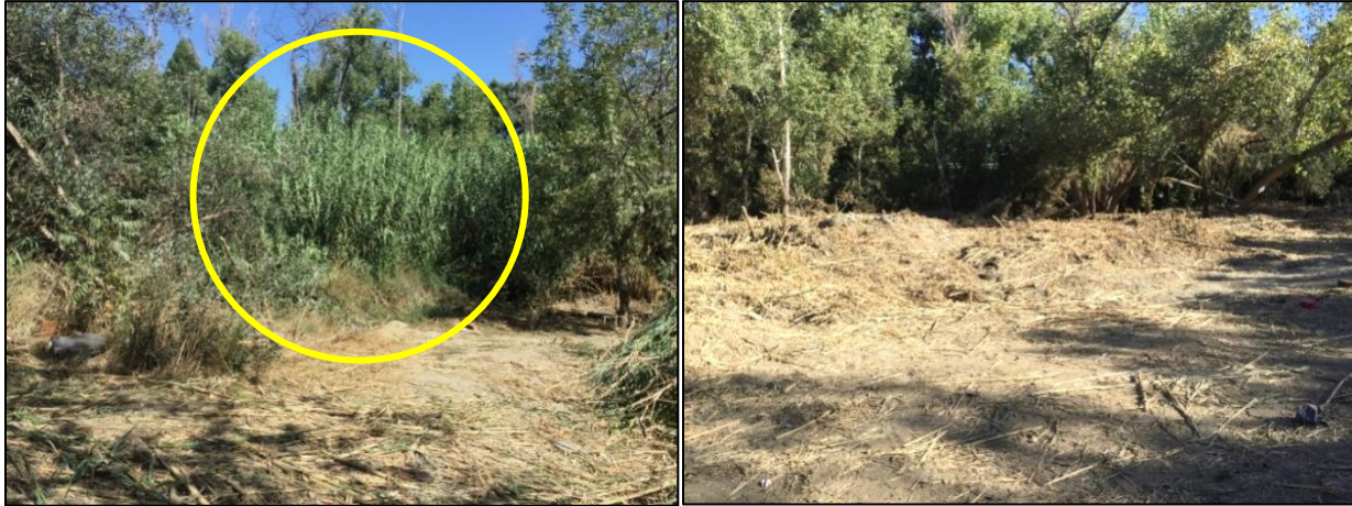
Before and after photo of Arundo removal (plant is inside the yellow circle).
