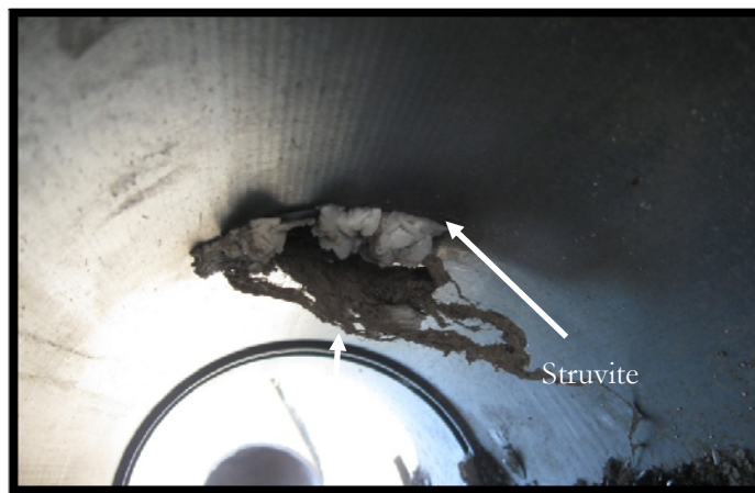
Figure 4-5. Inside of HDPE pipe found at the sludge lagoons where struvite has formed at the intake portion of a tee.
