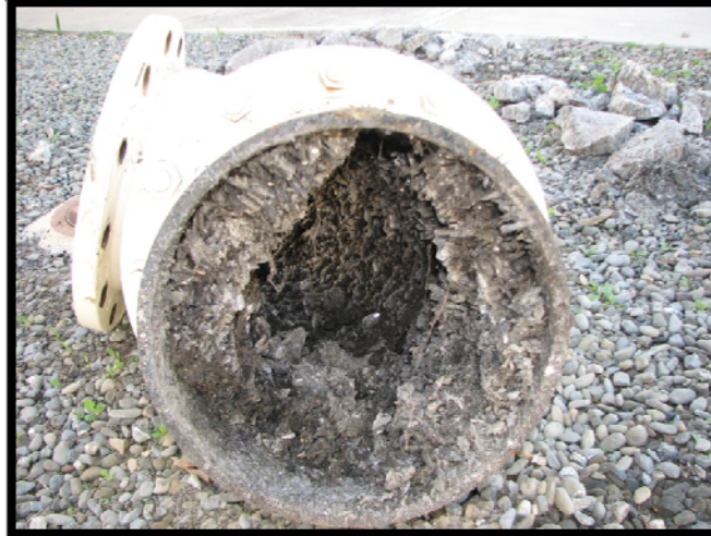
Figure 4-3. Struvite formation in the digester recirculation piping at the WPCP.
