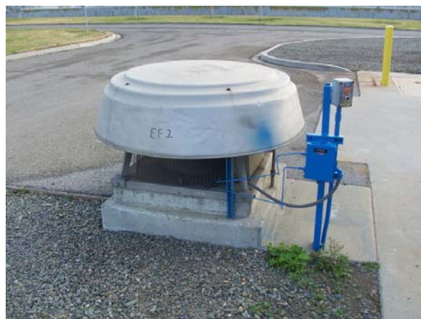
Figure 4-2. Typical exhaust fan (EF-2 shown)
