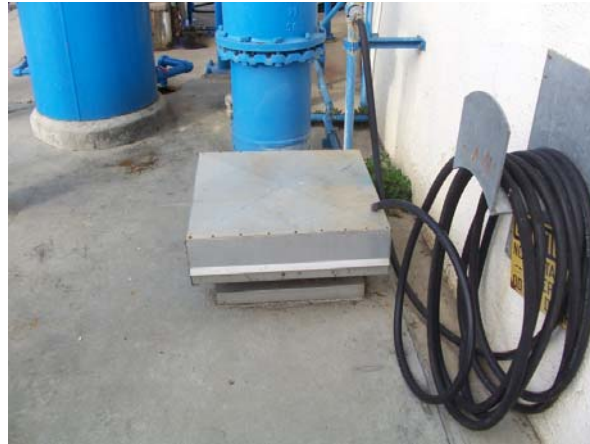
Figure 4-3. Poor intake hood location – IH-21-1 too close to Digester 15 (IH-21-2 and Digester 16 similar)
