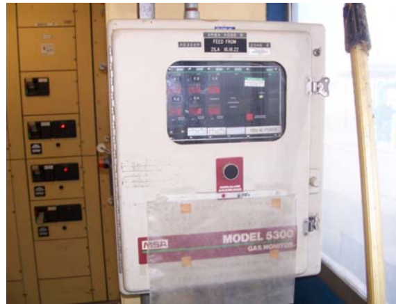
Figure 4-4. Gas detection system panel
