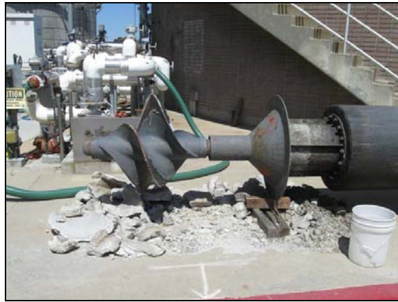
Figure 4-10. Draft tube mixer removed from DSRSD digester showing struvite that was removed.
