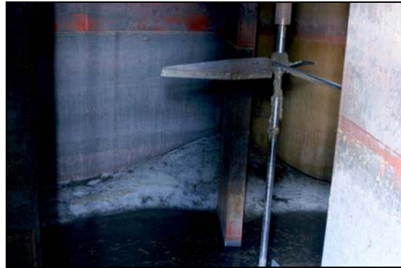
Figure 4-12. Inside of a digester at Clean Water Services in Durham, Oregon showing no struvite on the mixer and significant struvite accumulation in loose piles
