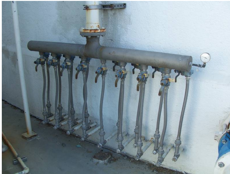
Figure 4-1. Gas piping at Digester 7
