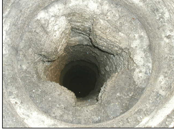
Figure 4-11. Inside of a draft tube coated with struvite after two years of operation from the Colorado Springs wastewater treatment plant.
