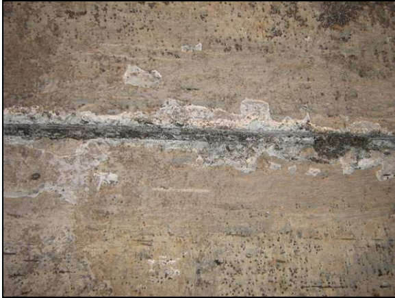
Photo 29. South wall joint with chips in concrete
