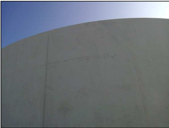
Photo 21. Exterior concrete, north wall with longitudinal crack in coating
