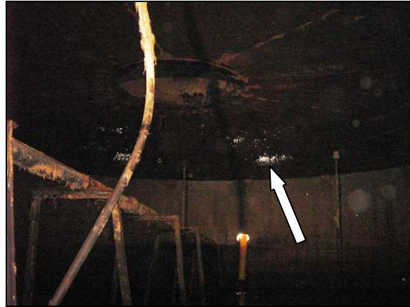
Photo 10. Steel roof interior surface with holes
