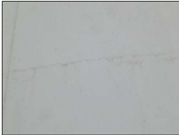
Photo 22. Exterior concrete wall with longitudinal crack in coating (detail)
