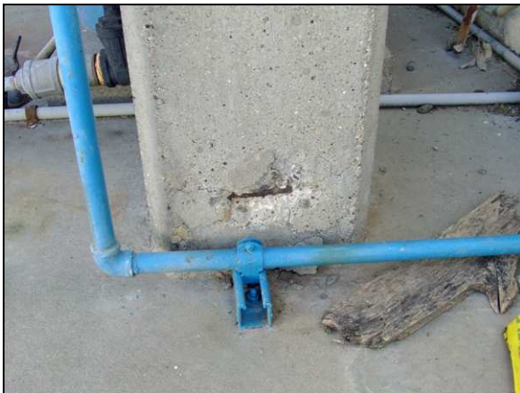
Photo 51. Spall in concrete support base
