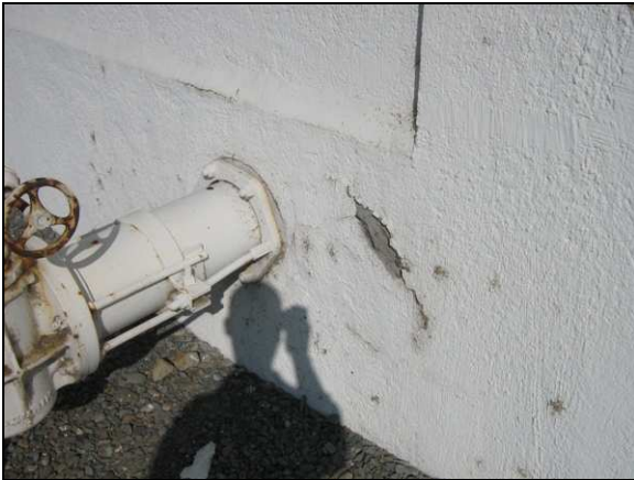
Photo 35. Medium-sized spall on south wall
