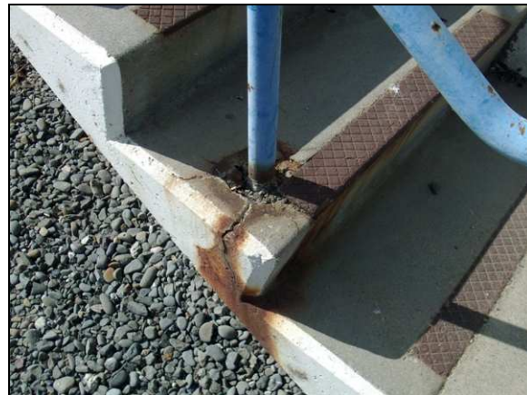
Photo 26. Fracture in concrete stairway due to corroding handrail (detail)
