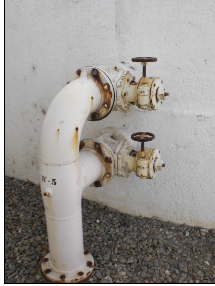
Photo 18. Superficial corrosion on digester gas piping
