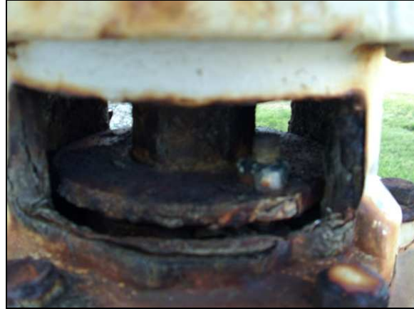
Photo 24. Corrosion on circulation pipe valve (detail)
