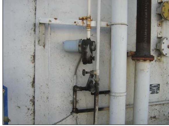
Photo 6. Miscellaneous actuators and valves with signs of leakage
