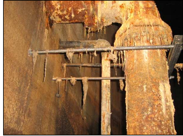
Photo 14. 8-inch cast iron sludge transfer piping with surface corrosion
