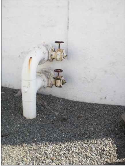
Photo 17. Superficial corrosion on circulation suction/discharge piping
