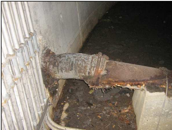
Photo 48. 8-inch cast iron sludge transfer pipe with surface corrosion
