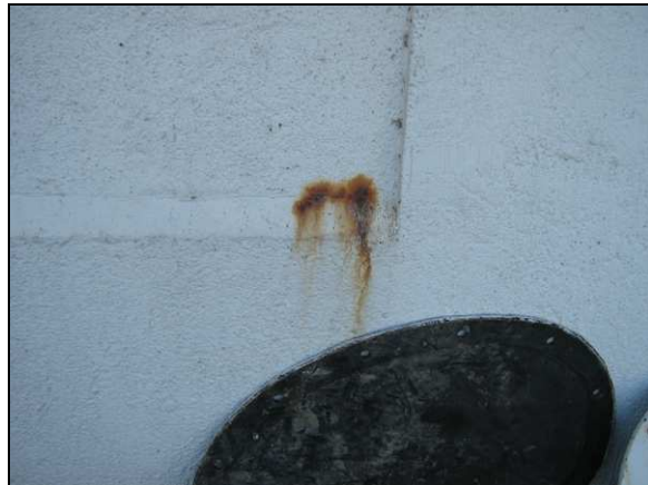
Photo 38. Exterior concrete wall with corrosion staining
