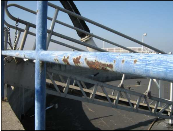
Photo 43. Corrosion on handrail system
