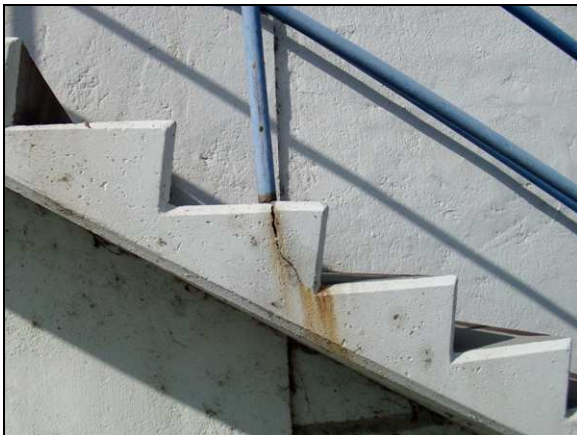
Photo 25. Fracture in concrete stairway due to corroding handrail
