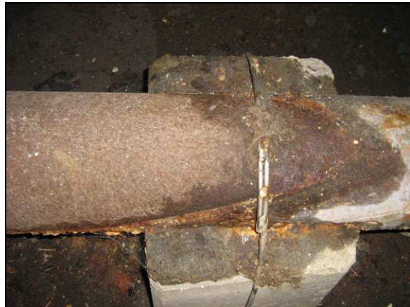
Photo 49. 8-inch cast iron sludge transfer pipe with surface corrosion (detail)
