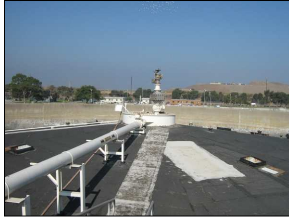
Photo 40. Digester gas piping in good condition
