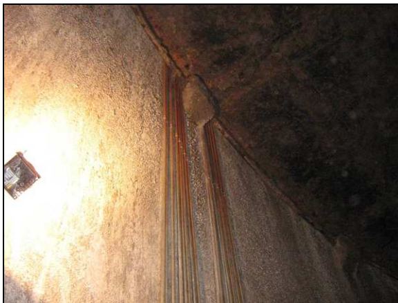
Photo 31. Roof with corroded conduits
