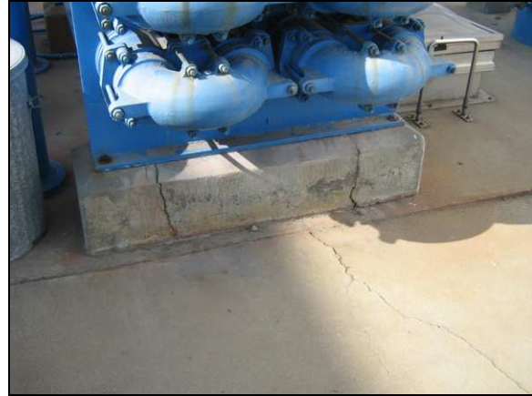
Photo 44. Multiple cracks have formed on the piping support
