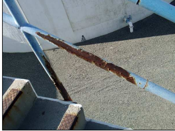
Photo 54. Surface corrosion area in the handrails
