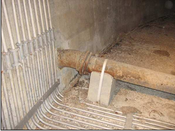
Photo 33. 8-inch cast iron sludge transfer pipe with surface corrosion
