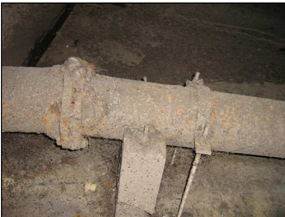
Photo 58. 8-inch cast iron sludge transfer pipe w/surface corrosion
