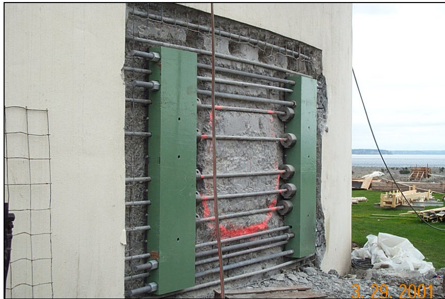
Figure 5-1. In a retrofit of an existing digester, a spreader bar installed to maintain support of digester post-tensioning around the location of the wall penetration.
