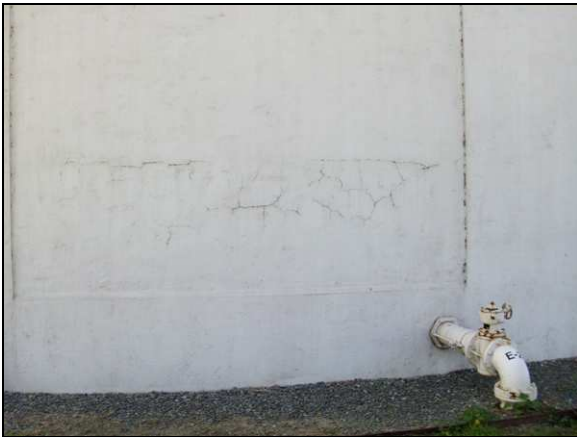
Photo 19. Exterior concrete, east wall with spider cracks in coating
