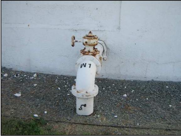
Photo 39. Corrosion on circulation pipe valve
