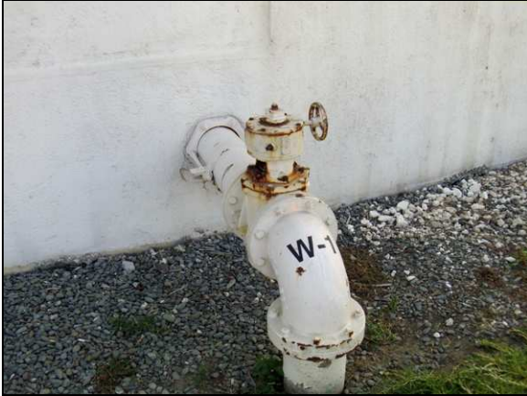
Photo 23. Corrosion on circulation pipe valve
