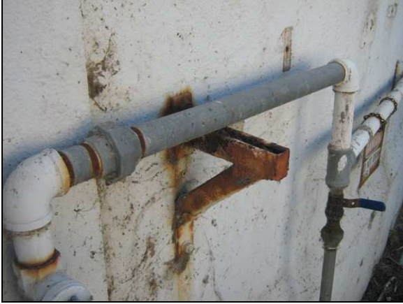
Photo 5. Miscellaneous pipe support bracket with surface corrosion
