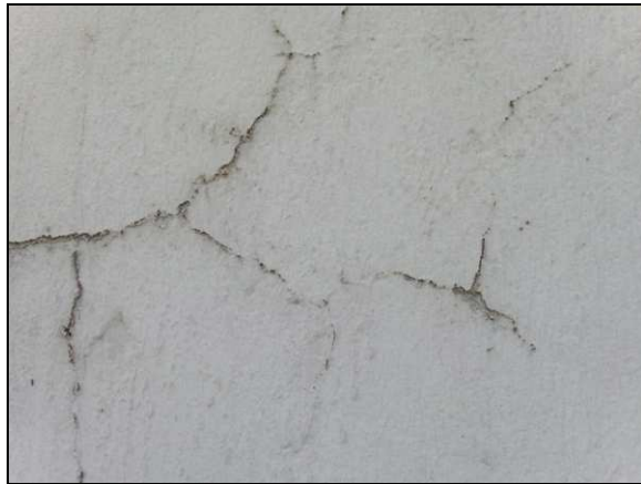
Photo 20. Exterior concrete, east wall with spider cracks in coating (detail)
