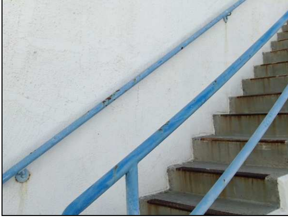
Photo 53. Surface corrosion spots in the handrails
