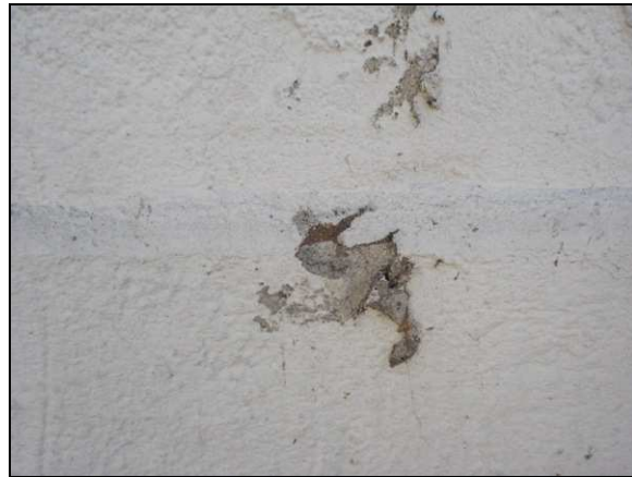
Photo 16. Exterior concrete, northeast wall with damage due to external impact
