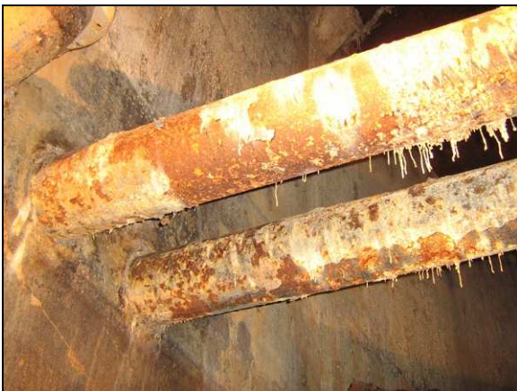
Photo 11. 8-inch cast iron circulation piping with surface corrosion
