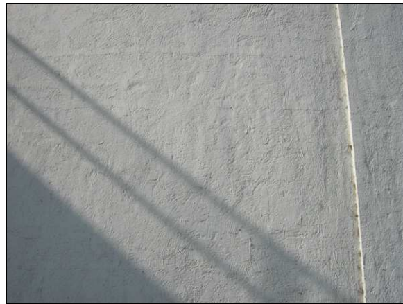
Photo 2. Exterior concrete wall showing patched spider cracks
