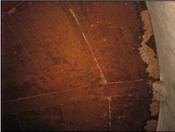
Photo 9. Steel roof interior surface with pitting
