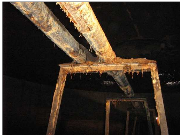
Photo 12. 8-inch cast iron circulation piping support brackets in good condition
