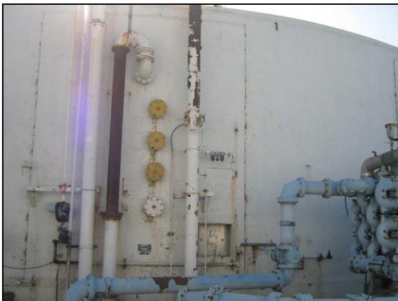
Photo 3. Corrosion on digester gas piping
