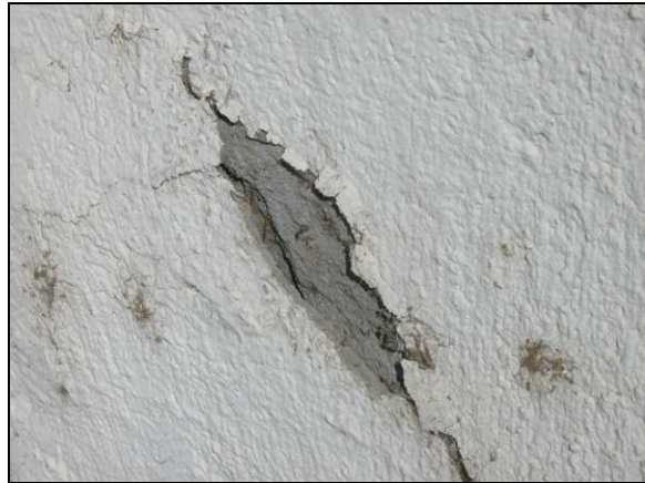
Photo 36. Medium-sized spall (detail)
