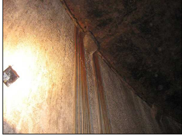
Photo 34. Conduits corroded near roof
