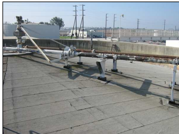
Photo 4. Corrosion on digester gas piping
