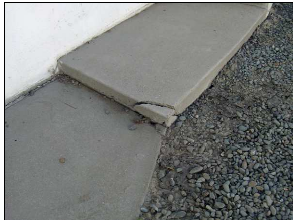
Photo 52. Fracture in concrete pathway
