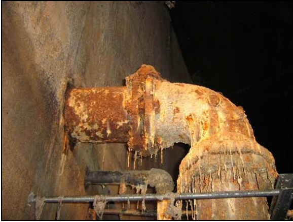
Photo 13. 8-inch cast iron sludge transfer piping with surface corrosion
