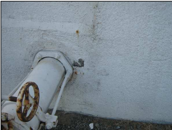
Photo 37. Small-sized spall near the E-2 inlet pipe on the east wall
