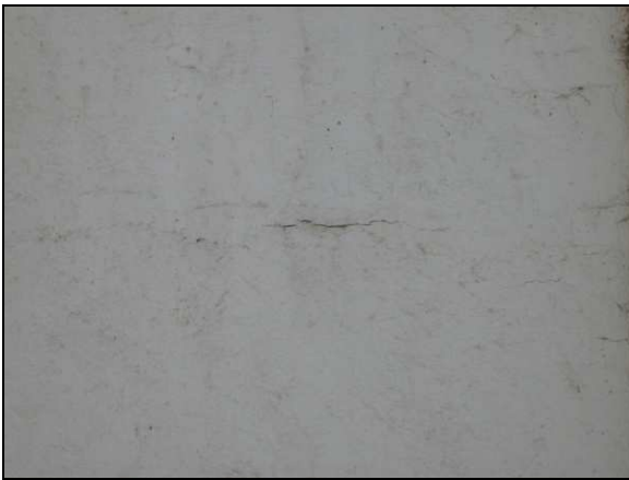
Photo 1. Exterior concrete, east wall with crack in Gunitite coating
