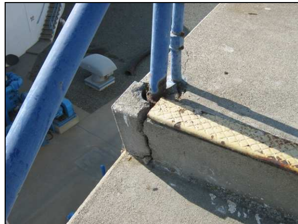
Photo 42. Fracture in the concrete stairway at the top of the stairway
