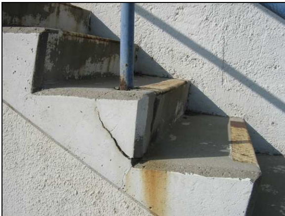
Photo 41. Fracture in the concrete stairway at the bottom of the stairway
