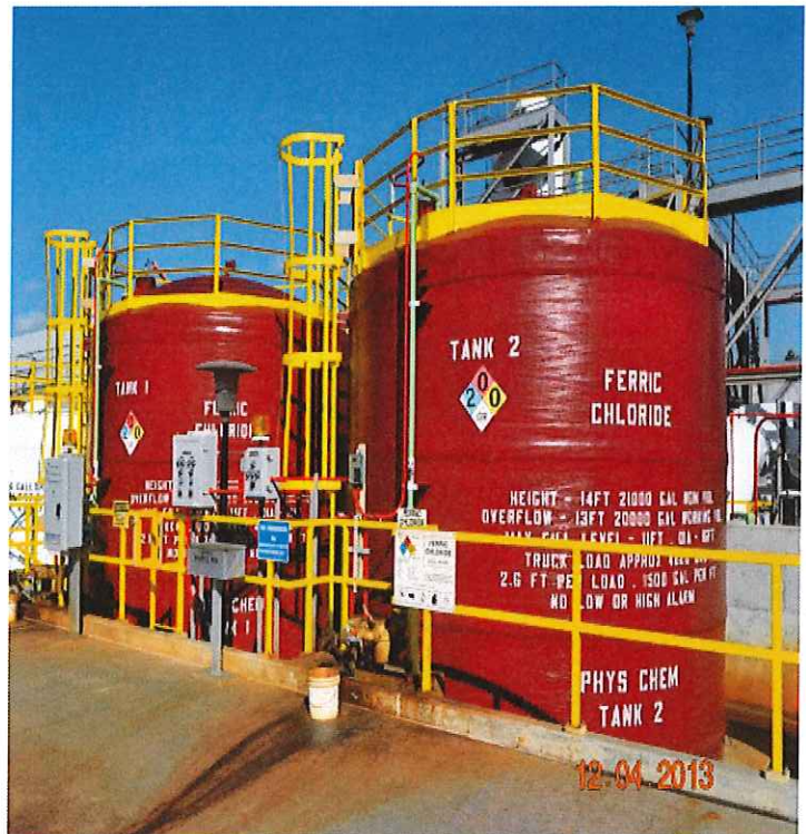
Figure 3— Example of a ferric chloride feed station similar in size to what is needed at the RWF. This installation is at Orange County Sanitation District's Plant No. 1, which treats an average flow of 96 mgd.
