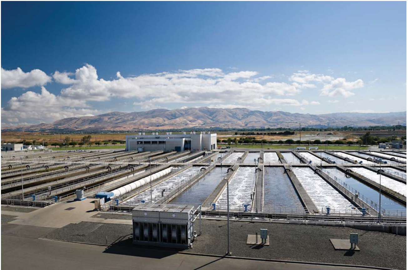
Eastward view of the secondary treatment tanks, which use bacteria to clean wastewater.
