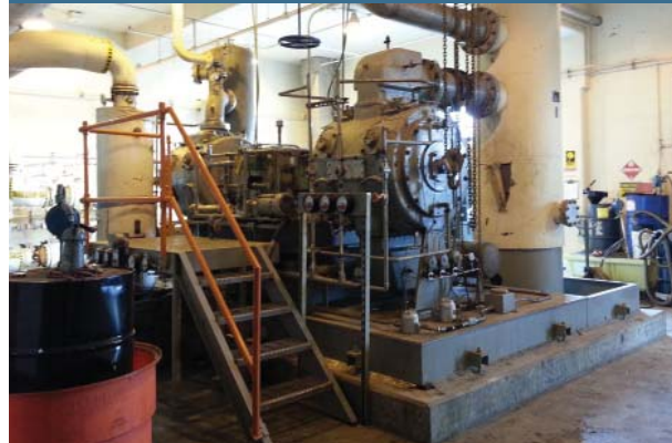
Existing digester gas compressor
