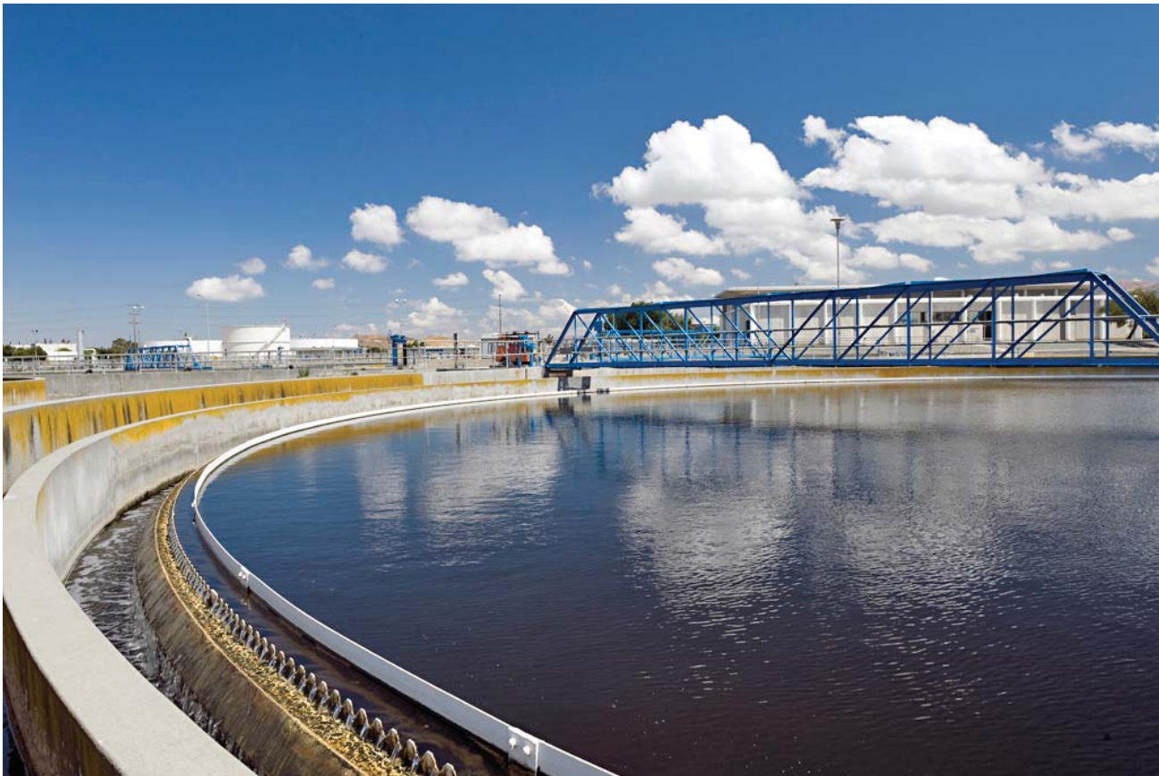
Clarifier tanks help settle solids during the secondary treatment process.
