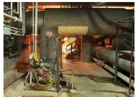
The Yard Piping Condition Assessment Plan will recommend an assessment approach for roughly 60,000 LF of process piping, much of which is underground.
