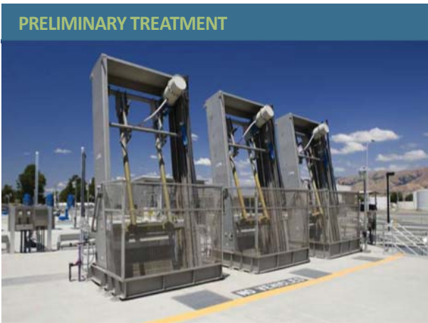
Headworks bar screens
