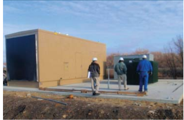
1.5 MW standby generator
