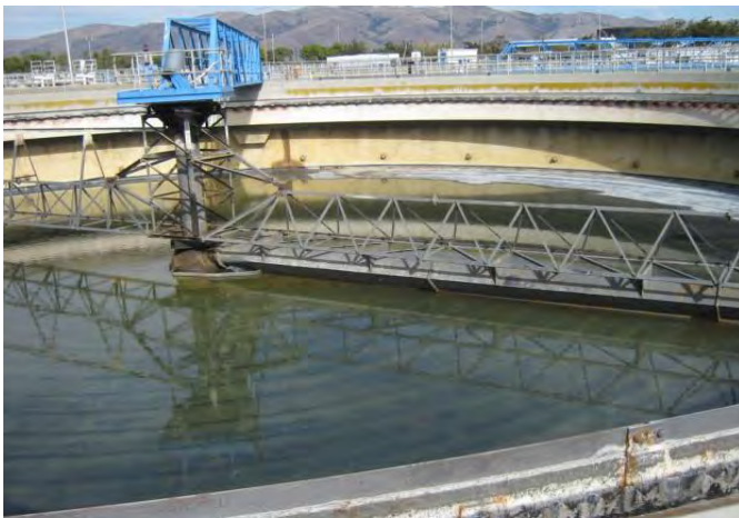
Figure 2— Picture of Clarifier interior and mechanism
