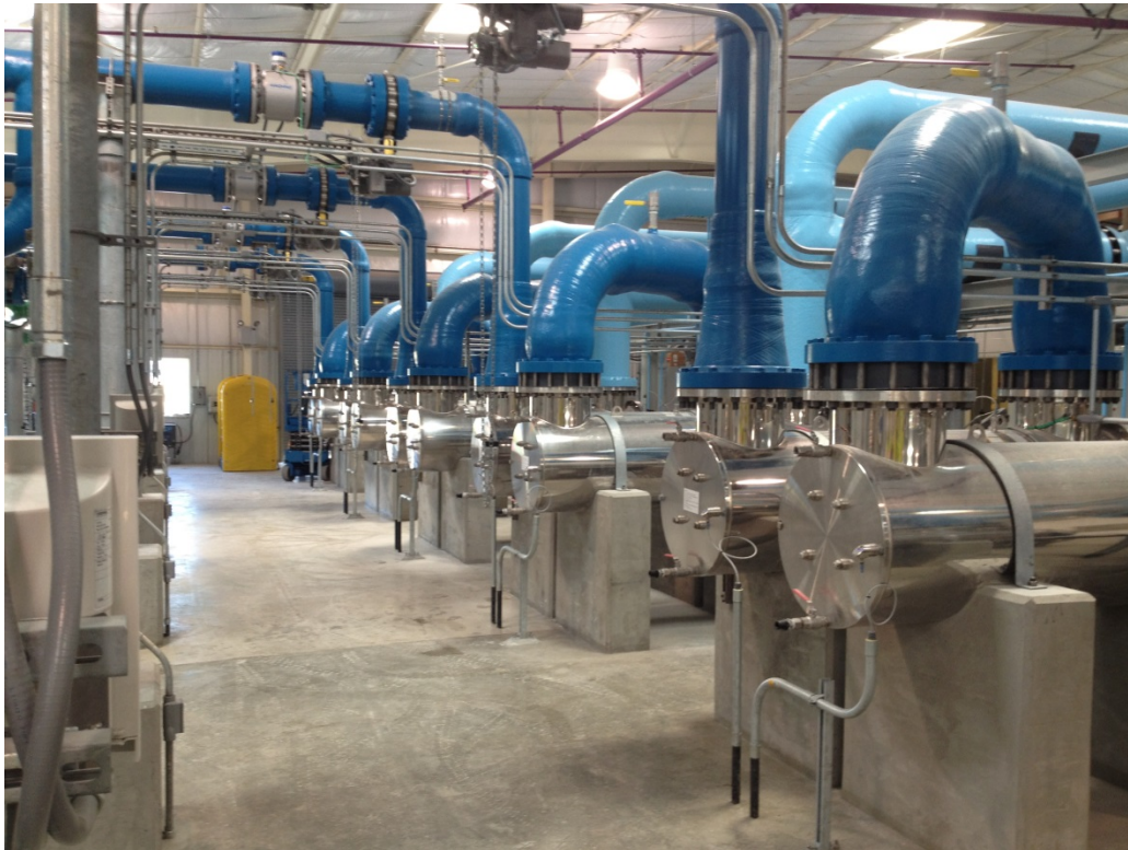
Figure 6-8: Pressurized UV System by Wedeco at the Existing SVAWPC
