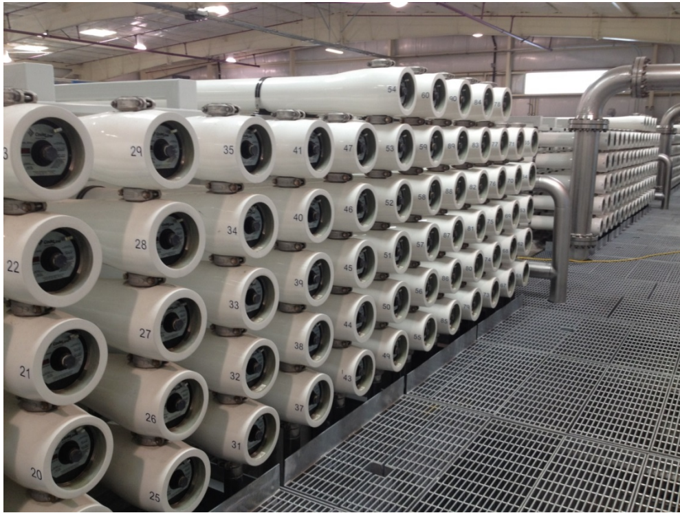
Figure 6-7: RO System at the Existing SVAWPC
