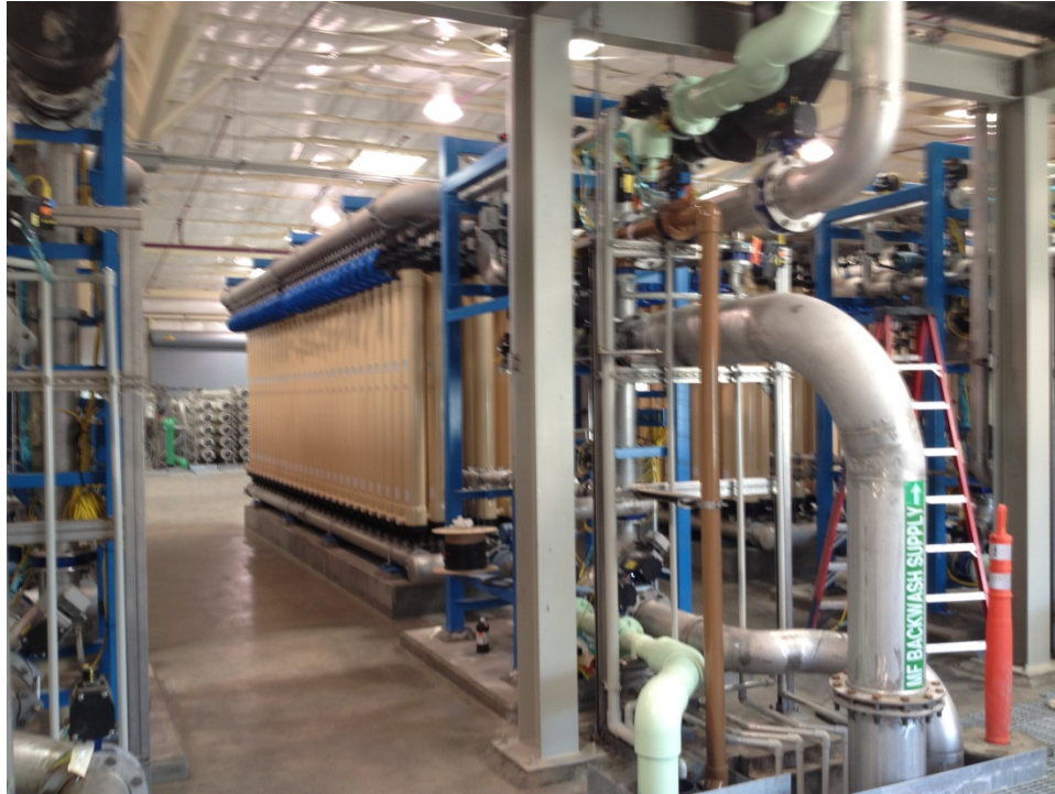
Figure 6-6: Pall MF System at the Existing SVAWPC
