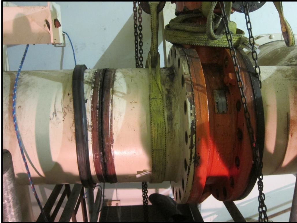
Figure 3: Typical Old Leaking Valve (30")
