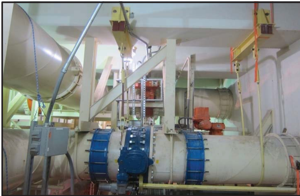
Figure 4: Typical New Valve (30")
